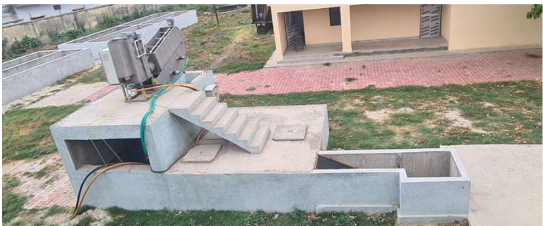
Image 10: Co-treatment unit for Faecal Sludge/Septage at STP
